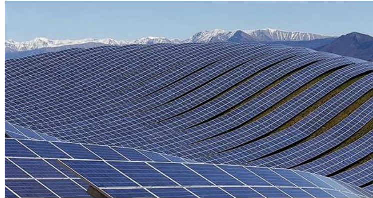
Solar PV farm, France
