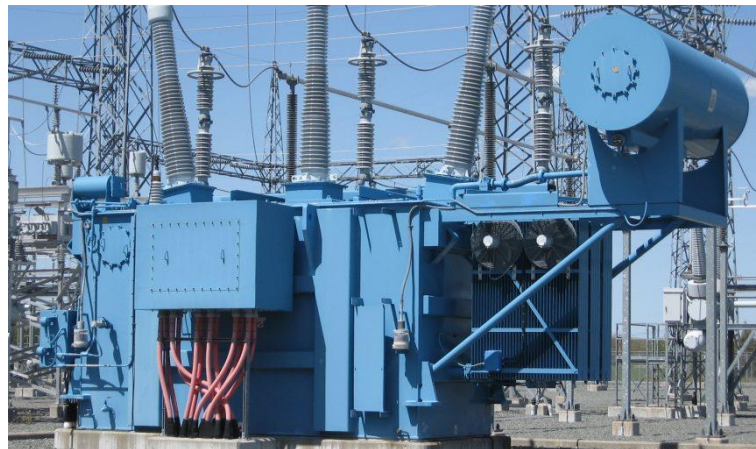
High voltage power transformer
