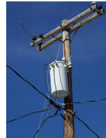
Local distribution transformer
